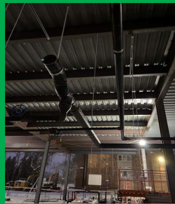
Temporary Steam Piping
